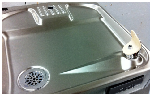
Exchange Bubbler hardware.
